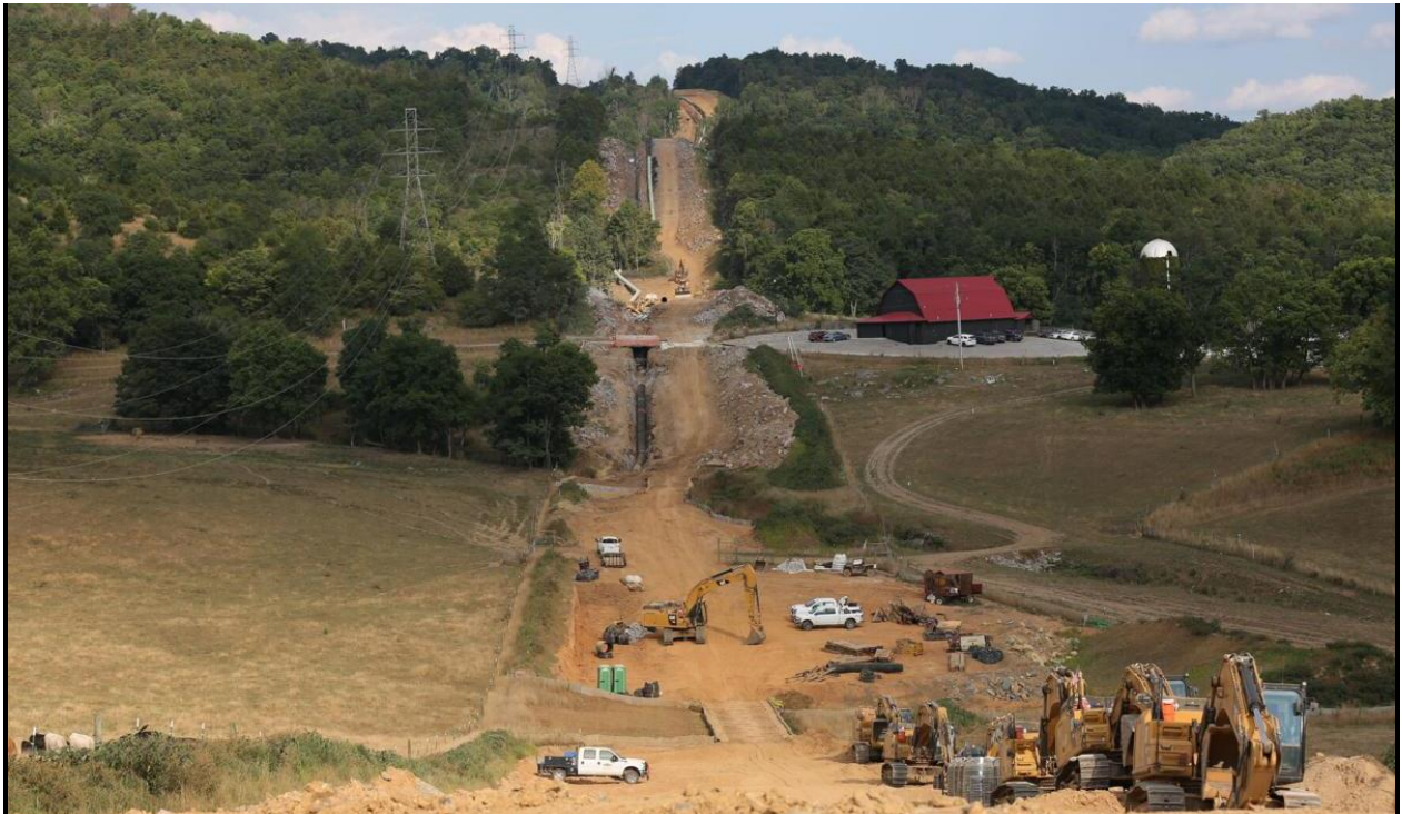
Construction of the Mountain Valley Pipeline comes through Doe Creek Farm in Giles County. HEATHER ROUSSEAU, The Roanoke Times
