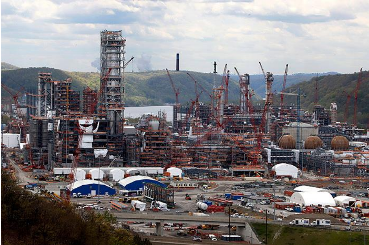
Construction on Shell Chemicals Beaver County ethane cracker plant in Potter Township, Pa. | Gene J Puskar/AP/Shutterstock
