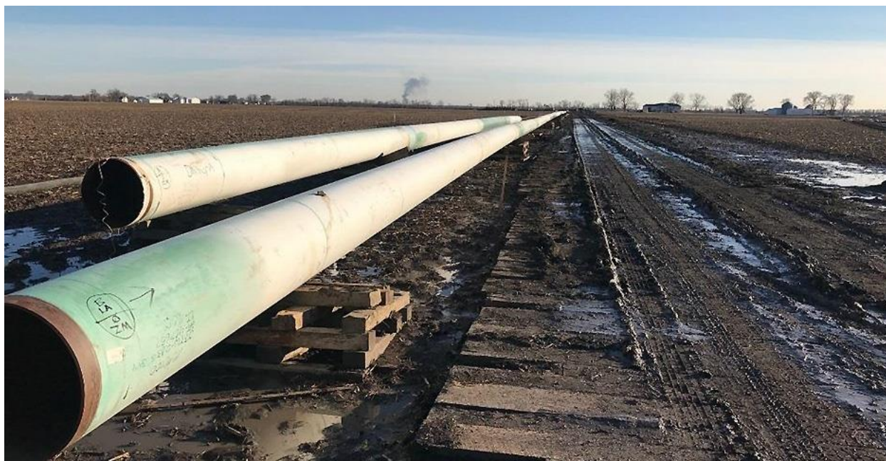
Pieces of the Spire STL natural gas pipeline awaiting construction are pictured. Federal Energy Regulatory Commission
