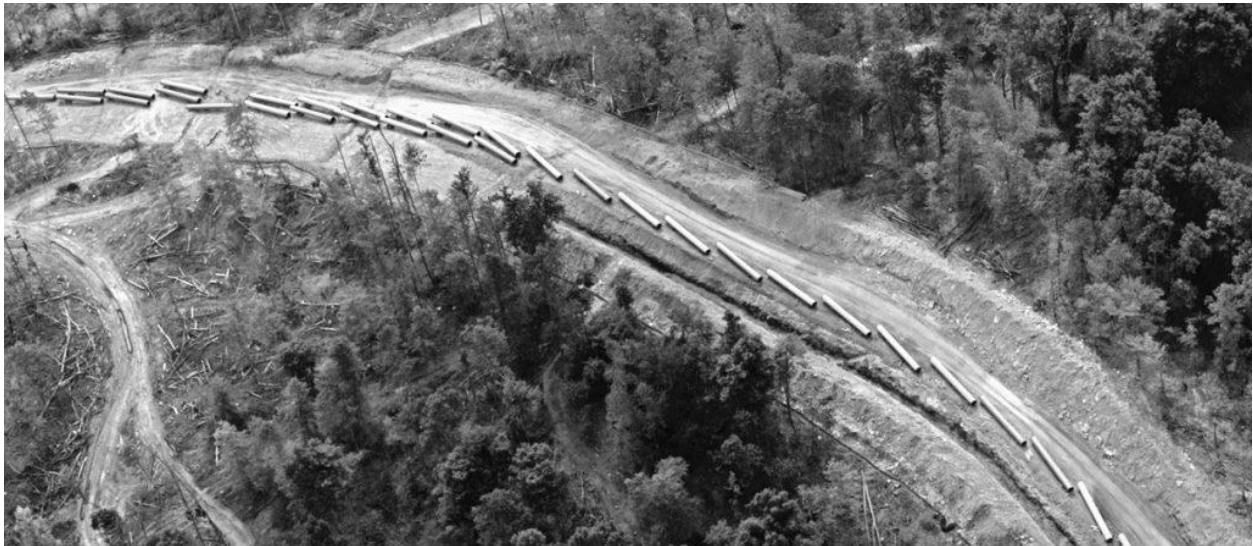
The Pipeline Air Force photographed construction in West Virginia. (Courtesy Dominion Pipeline Monitoring Coalition)
