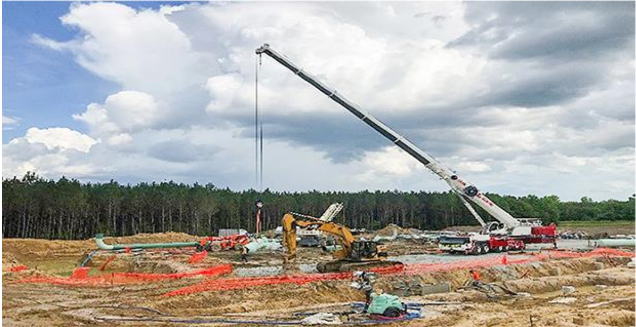
Construction crews working on an Atlantic Coast pipeline metering station in North Carolina. Atlantic Coast Pipeline LLC
