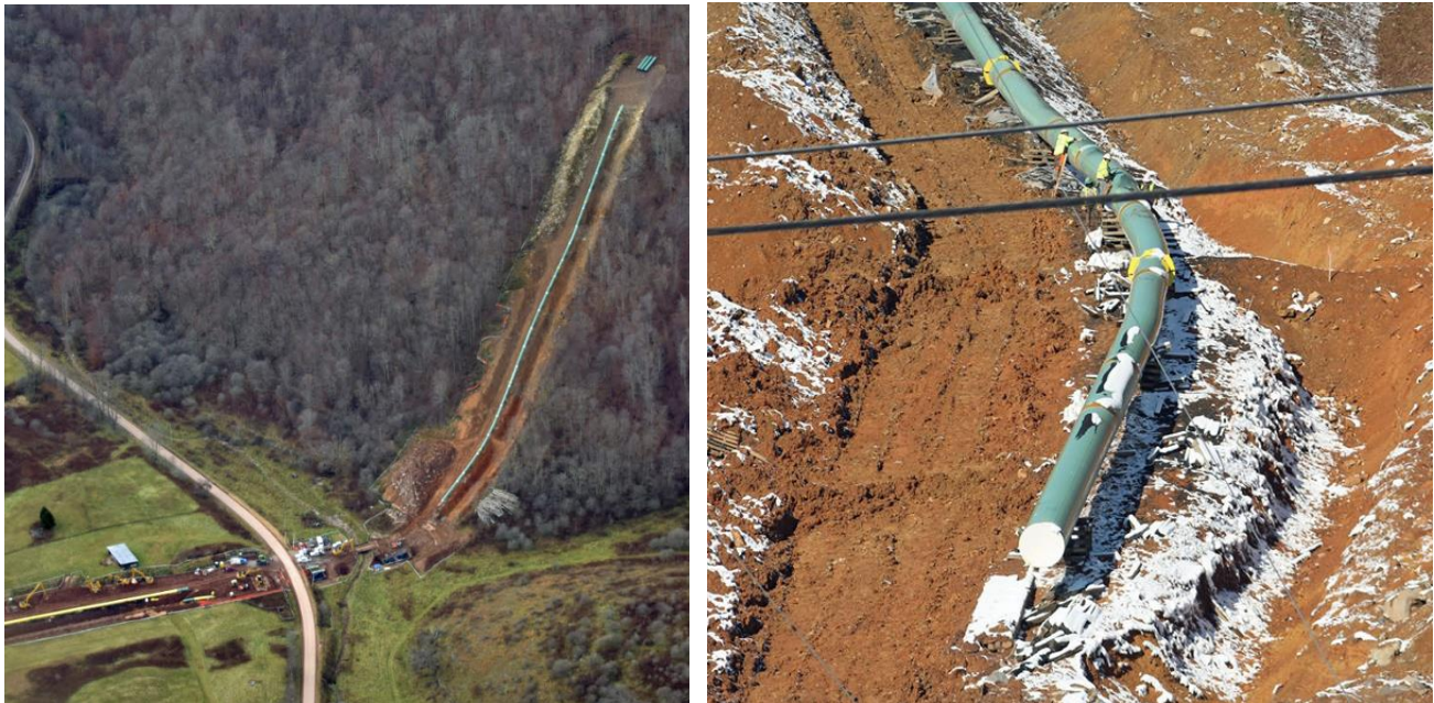
Above left: Pipeline Air Force photo of ACP construction in Dry Branch and Middle Mountain area in Pocahontas County. Above right: Citizen volunteer observer photo of ACP construction on Middle Mountain in Pocahontas County. In both instances, water bars are not installed as required for steep slope construction.
