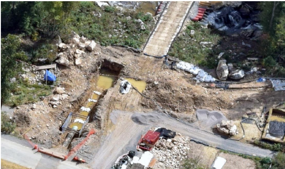
Pipeline construction at Grassy Run in Upshur County, West Virginia. An example of the kind of photos that photo reviewers would be examining.
