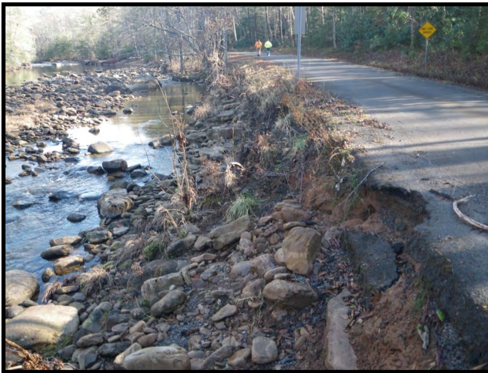
Figure 1. Williams River Road near MP 10.7, photo taken 11/30/2017
